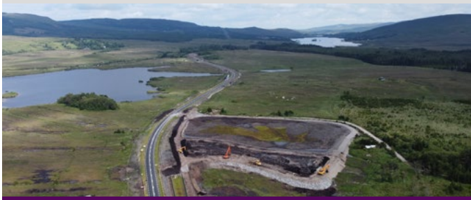
Peat deposition area constructed as part of N59 project near Maam Cross, Co. Galway.
