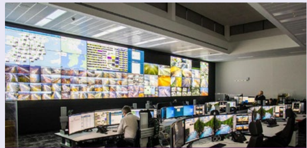
The main control room in the motorway operations control centre.
